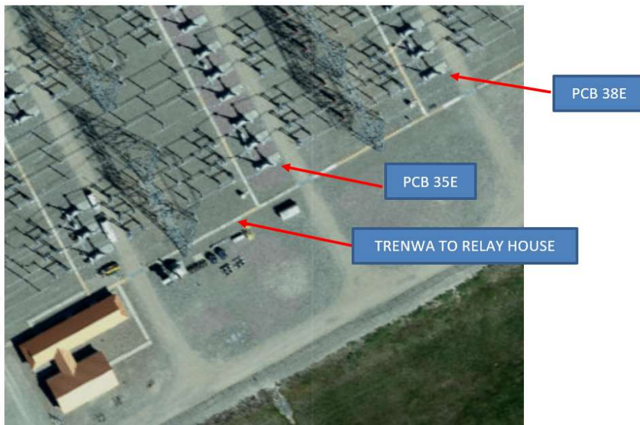
Figure 6. Location of tie and bus breakers and the trench to the control house
