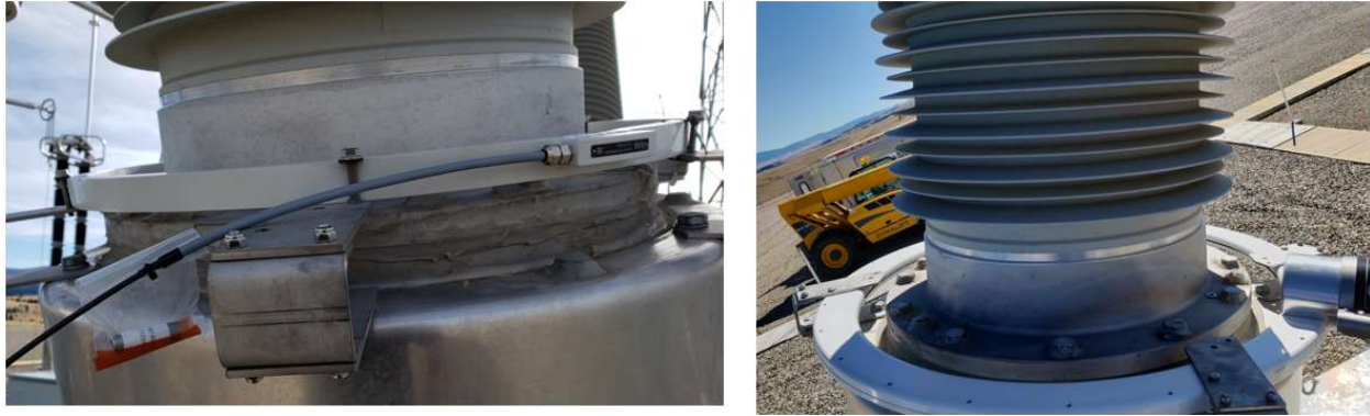
Figure 9. FOCS devices from two vendors installed on a 500kV circuit breaker.
