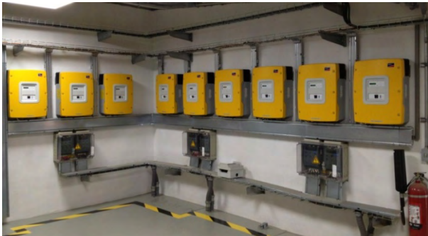
Fig. 5. Battery system inverters installed in the inverter room of the Guásimas del Metate solar farm. (Photo courtesy of Greenergy.)
