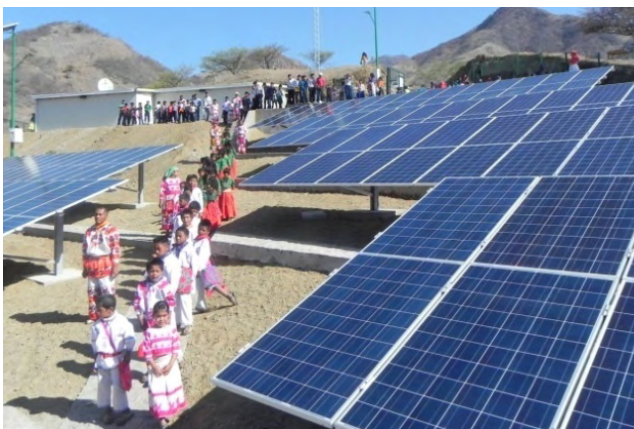
Fig. 3. Solar panels installed at the Guásimas del Metate solar farm. (Photo courtesy of Greenergy.)
