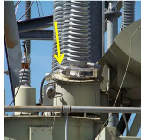
Figure 2 – Open Phase Field Testing on a 238 kV Wye-Wye Transformer
