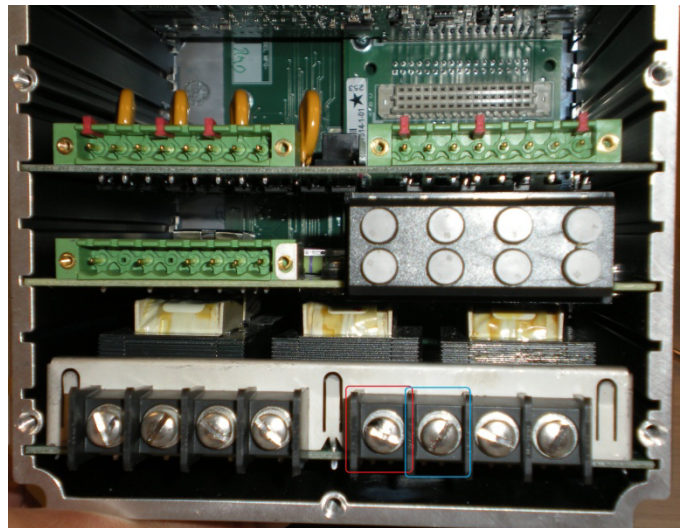
Fig. 25. Relay Rear Panel Removed to Expose Inside
