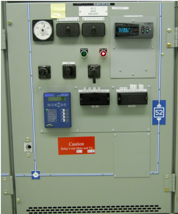
Fig. 9. Switchgear Breaker, Relay, and Controls
