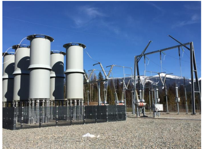
Figure 1 – Avista's NRR Reactor Banks (one bank shown)
