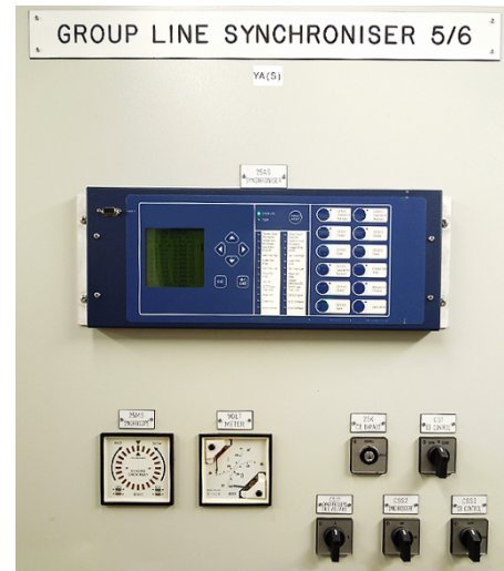
Fig. 7. Example Line-Synchronising Panel
