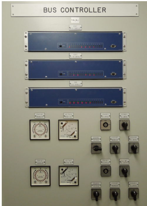
Fig. 6. Example Bus-Synchronising Panel
