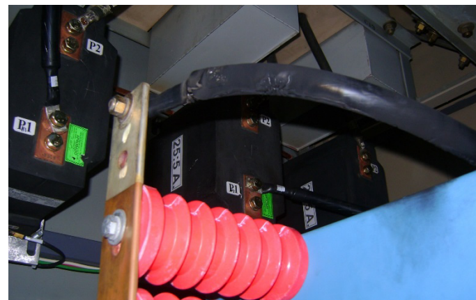
Fig. 30. Fast tripping for a cable failure at the generator bus limited its damage; the cable repair cost was minimal.
