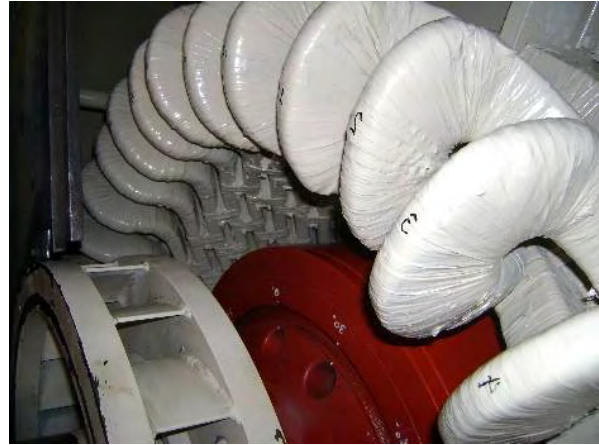
Fig. 6. A 26.6 MVA, 13.8 kV, direct air-cooled turbogenerator end.
