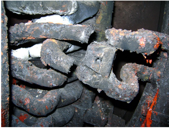
Fig. 20. Another view of the generator damage after phase-to-ground and phase-to-phase faults at different winding locations.
