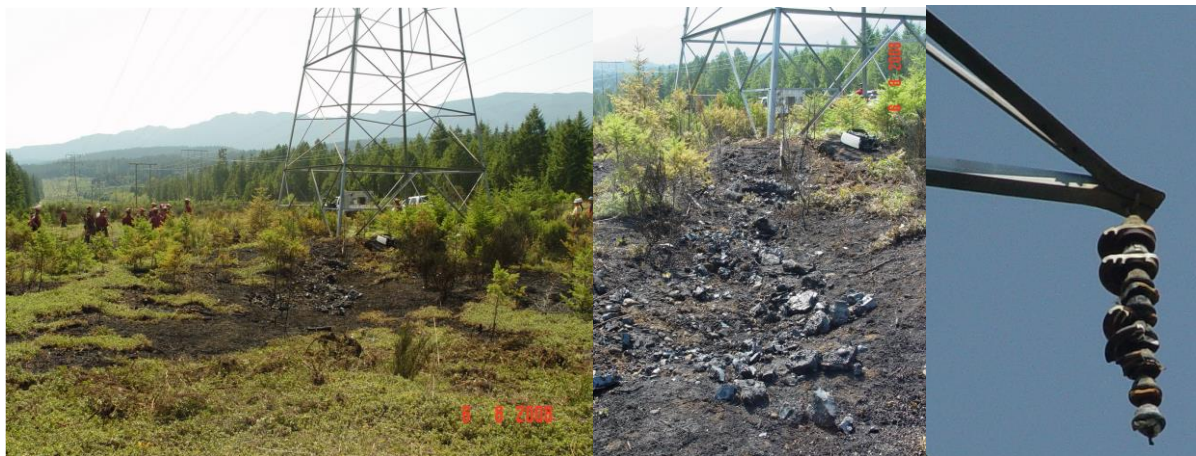
Figure 3 Aftermath of a 200-ohm 138 kV line 1LG fault
