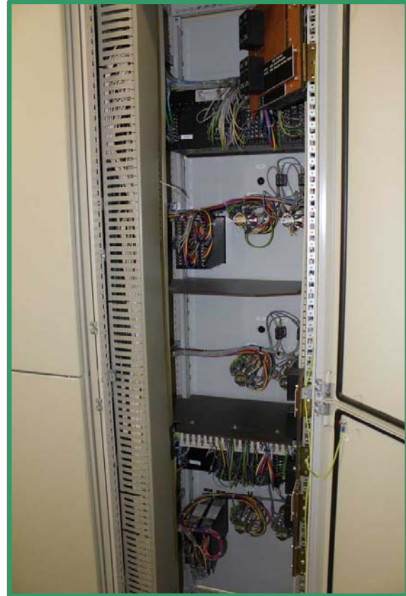
Figure 10: Rear view of traditionally wired panel
