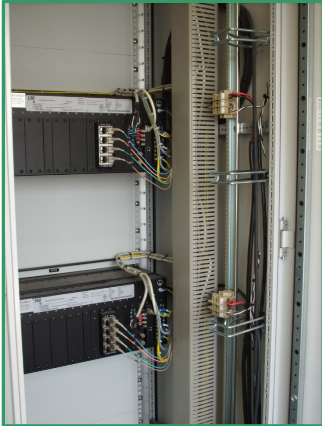
Figure 9: Rear view of relay panel
