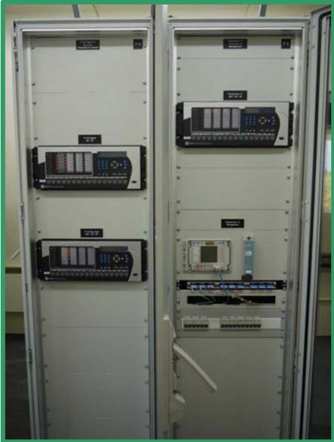
Figure 8: Front view of relay panels
