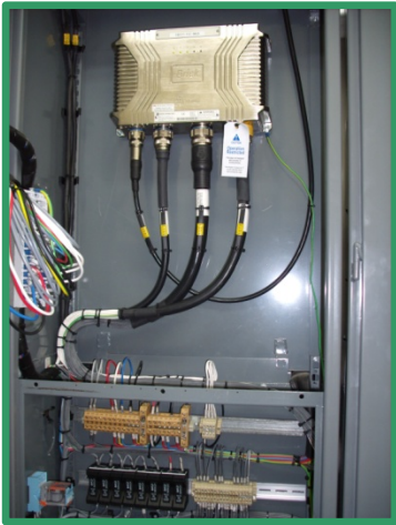
Figure 6: PIU mounted in 11 kV switchgear
