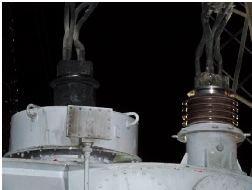
Fig. 12. 9/22/2010, Location 1: Tertiary bushing failure
