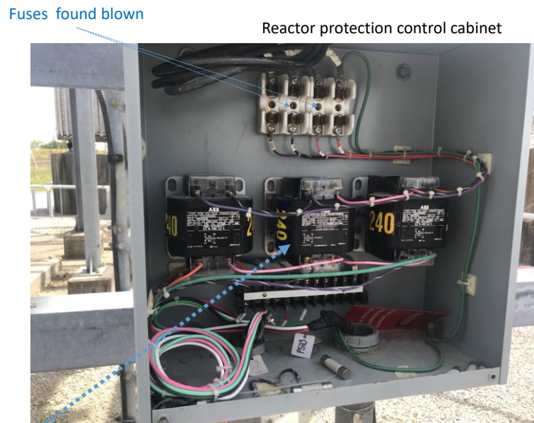
B-phase aux VT shorted primary-to-secondary
