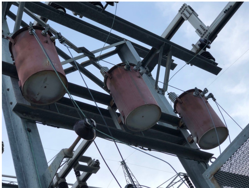
Fig. 24. 4/30/2019 Location 4 - Tertiary bus voltage transformers
