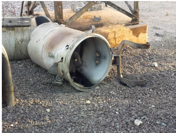
Fig. 17. Location 2 6/15/2015 - Tertiary VT failure
