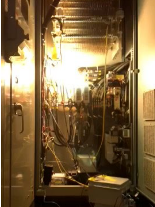
Fig. 8. Contact arcing during a poorly timed field breaker closure.
