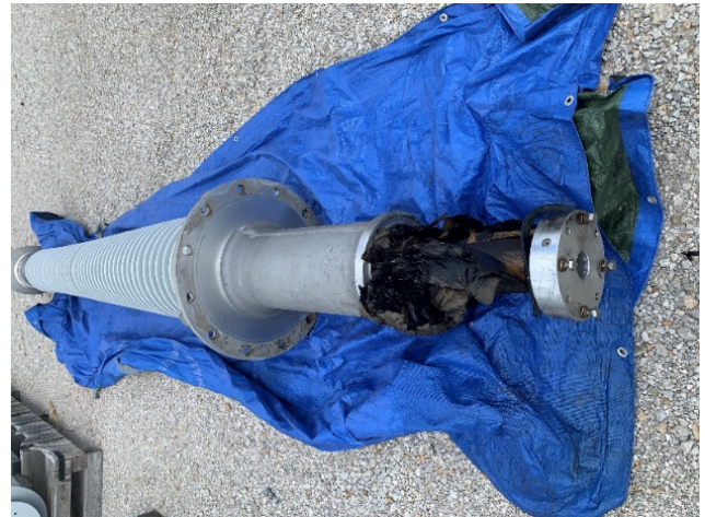
Fig. 22. Removed damaged reactor bushing at Romney.
