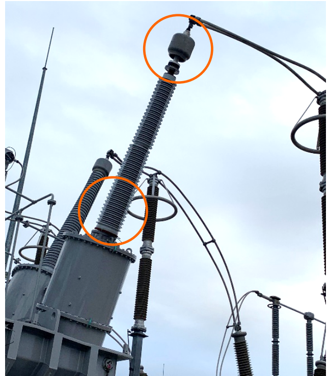
Fig. 21. Damaged reactor bushing at Romney.
