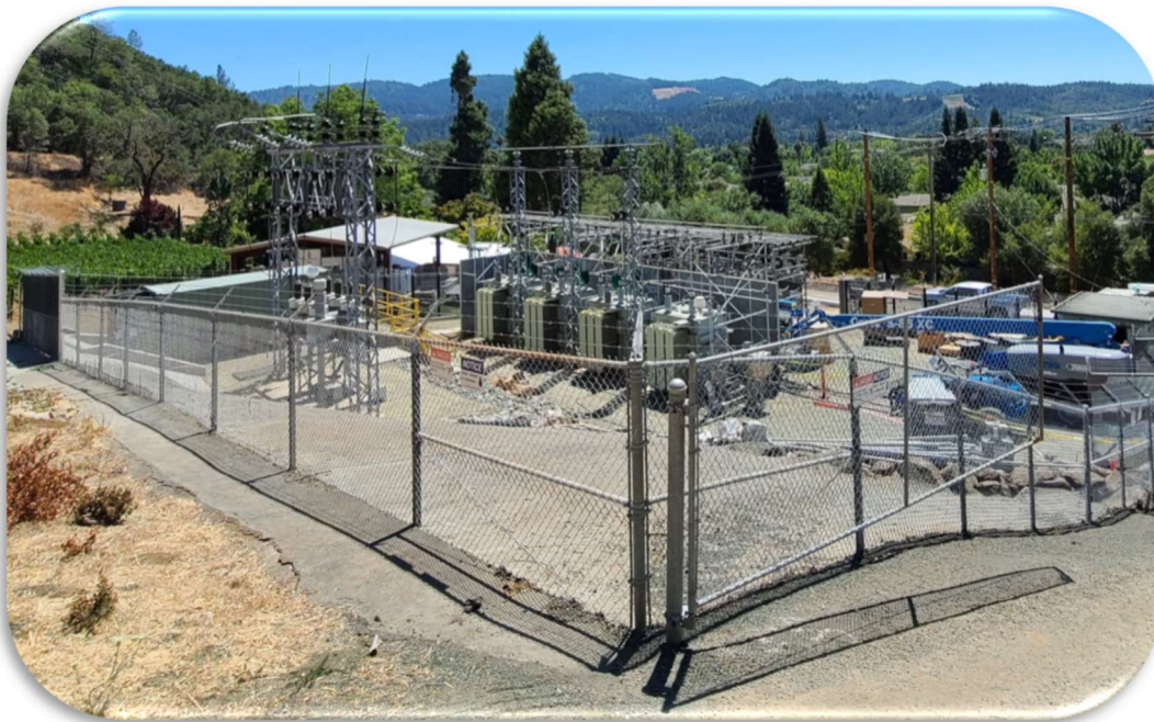
Figure 2 GFN pilot substation in Napa Valley California
