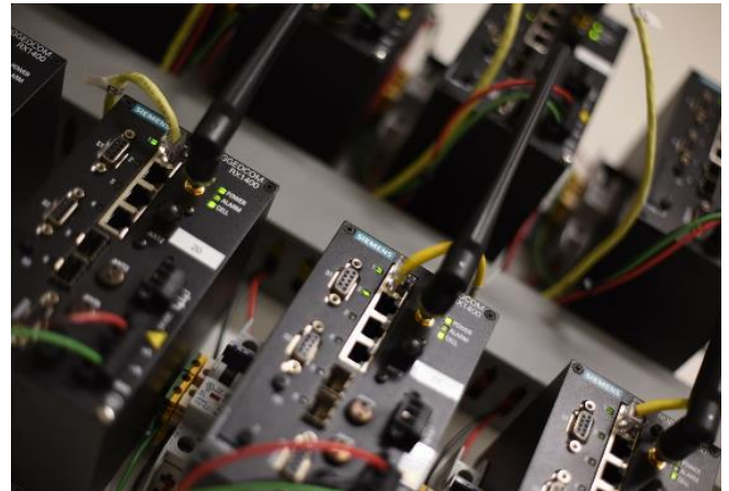
Fig.11. Communication infrastructure with 23 RX1400 Modems
