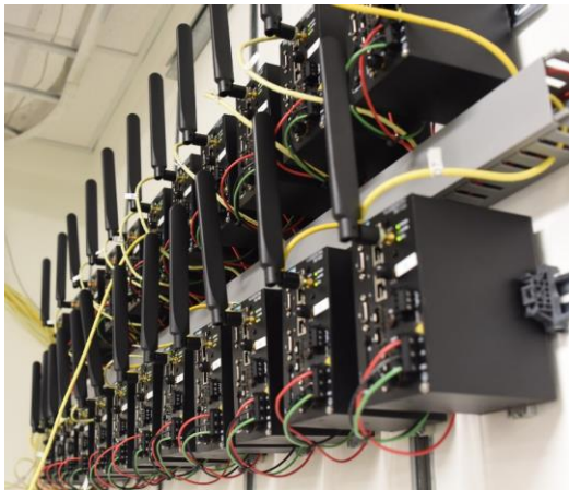
Fig. 10. Communication infrastructure with 23 RX1400 Modems
