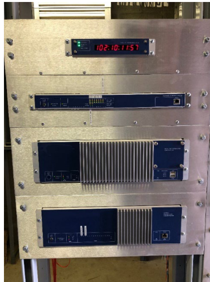
Figure 5: FCP substation IEDs
