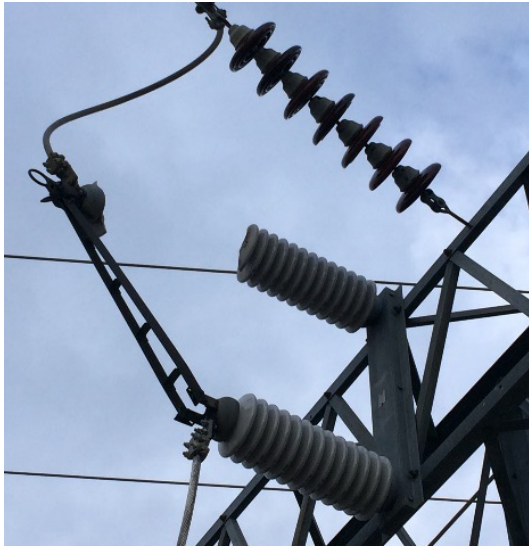
Fig. 5. First fault on A-phase of Switch S11
