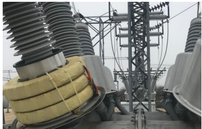
Fig. 11. Cover of Pole 1 removed
