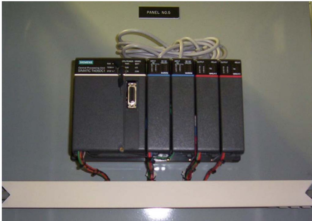
Figure 10 - Close up view of programmable logic controller in rear of panel.
