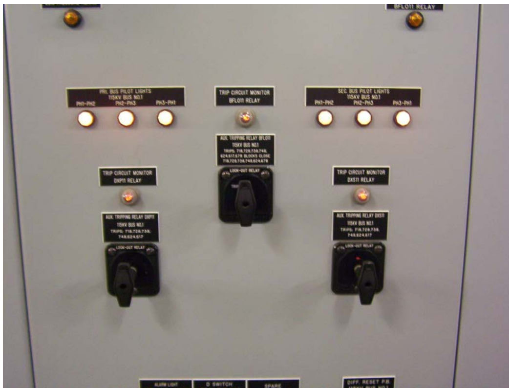
Figure 11 - Close up view of auxiliary tripping relays, manual reset breaker failure relay in the middle and the electric reset lockout relays on the outside.
