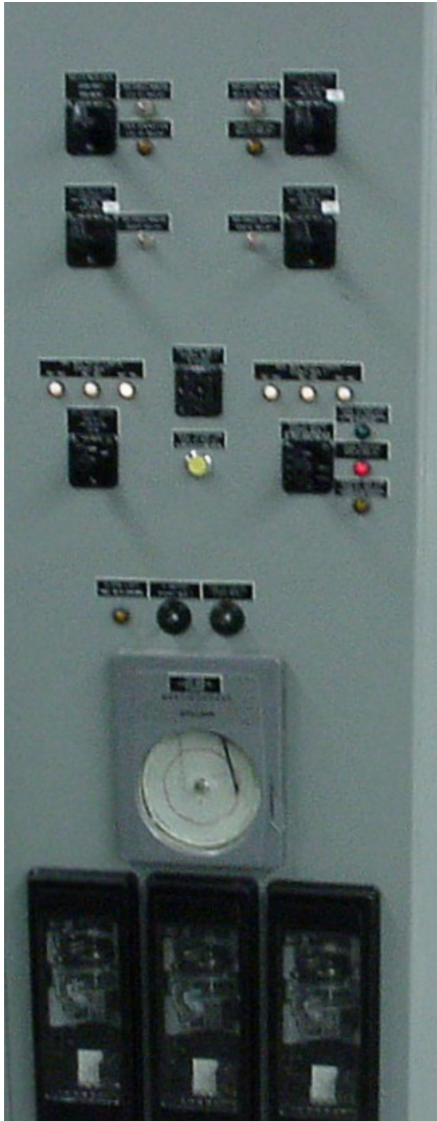
Figure 6 - Second Generation Stepper Switch Panel
