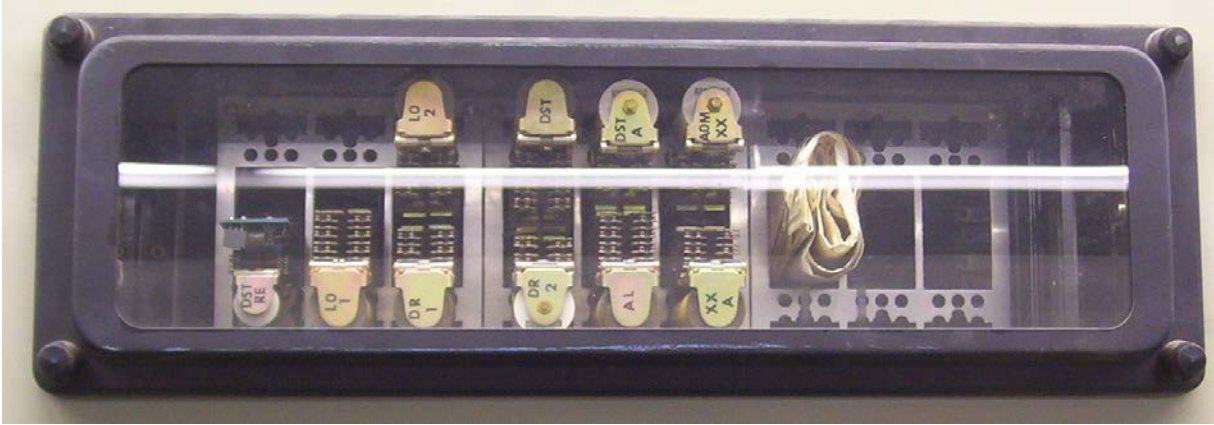
Figure 4 - Close up view of automatic box showing telephone relays.
