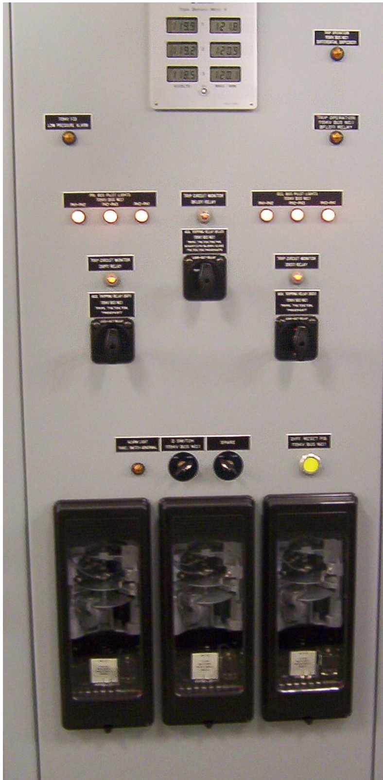
Figure 8 - Third Generation PLC Panel with PLC mounted in back
