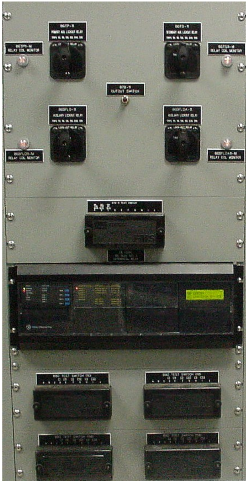
Figure 12 - Fourth Generation Microprocessor Relay Panel with the lockout relays on top (two manual reset for breaker failure and two electric reset for differential tripping), the microprocessor low impedance bus protection relay and the test switches at the bottom.
