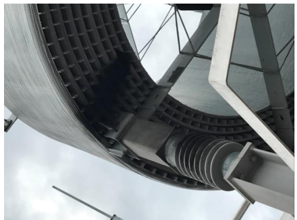
Figure 7: C-Phase faulty reactor following the 11/12/2017 event
