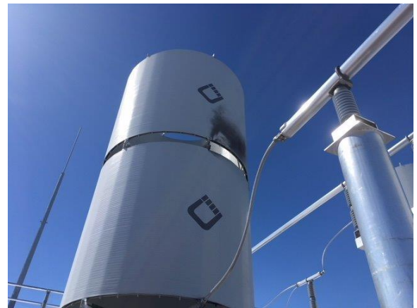
Figure 13: A-Phase faulty reactor following the 4/14/2018 event
