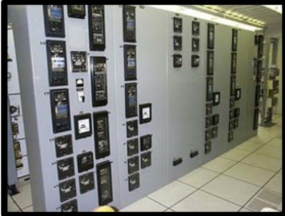
Figure 8 - Typical EM Relay Panels
