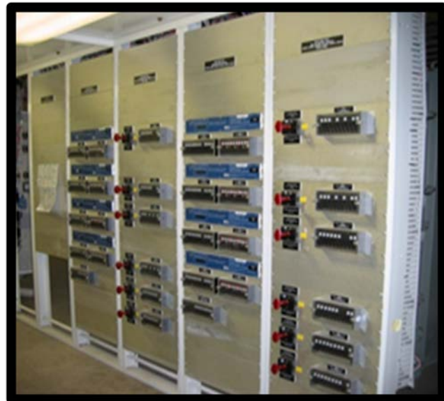
Figure 10 - Typical MP Relay Panels
