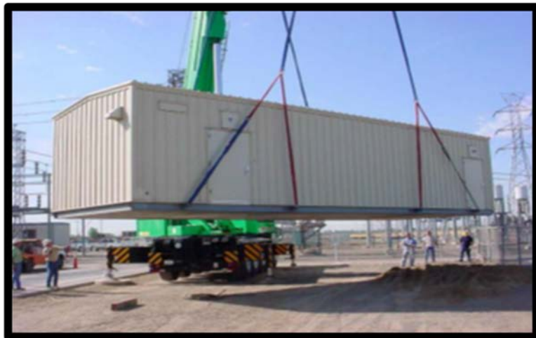
Figure 5 - Drop-in Control Building
