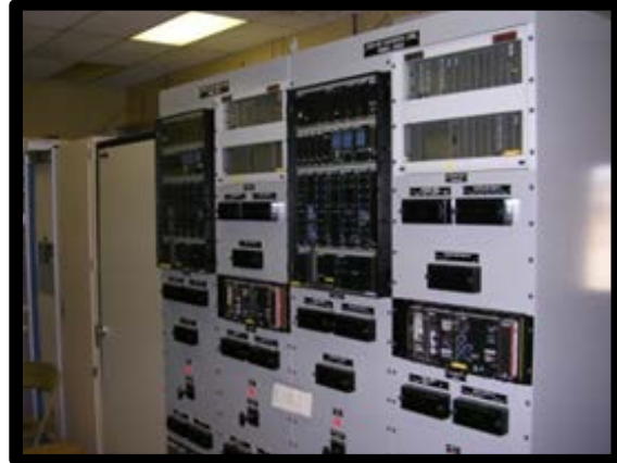
Figure 9 - Typical SS Relay Panels
