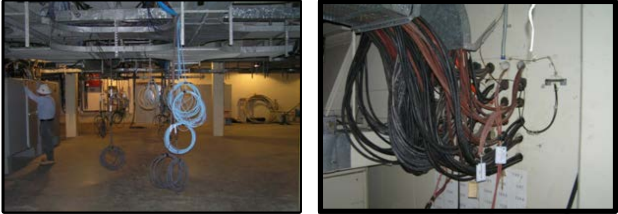
Figure 7 – Newer switchyard wiring enters via the basement of control building.
