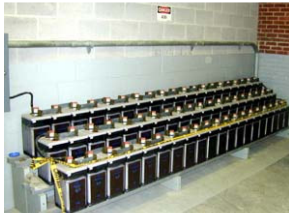
Fig. 3: Banks of batteries
