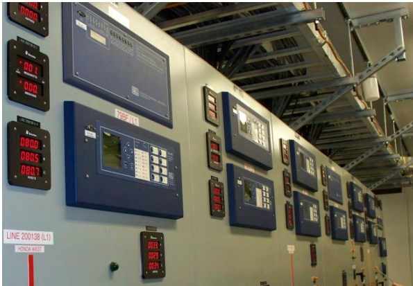
Fig. 1. Relays With Synchrophasors in Protection Panels
