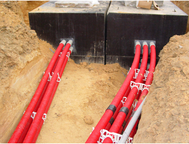
Fig. 2. Direct-buried conduit for fiber link and high-voltage cables
