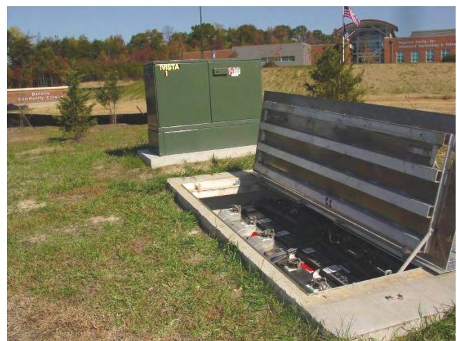
Fig. 6. High-speed fault-clearing system installed at Cyber Park
