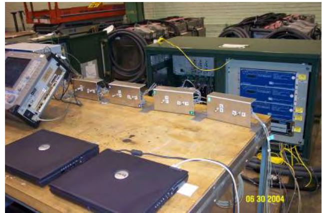
Fig. 5. Factory testing of protection schemes and communications
