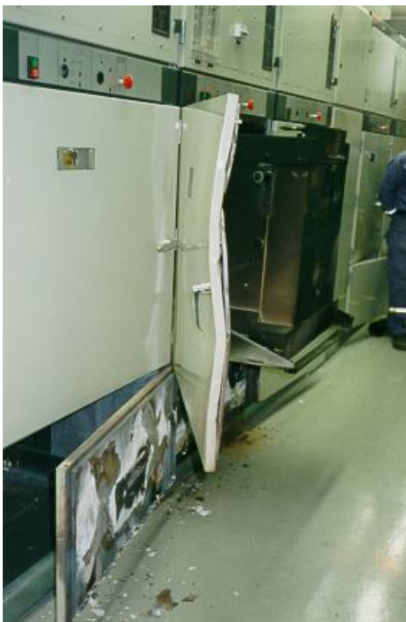
Figure 1: A cubicle damaged by arc short-circuit.
