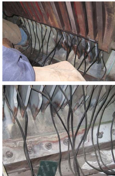
Figure 19. Photo of secondary flashover result with very fast tripping....minimal damage
