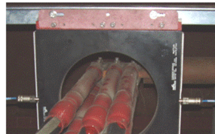
(a) Rogowski Coil monitors six conductors
