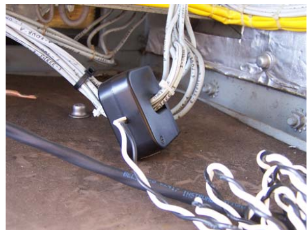
Figure 14 - An Actual Installation of Open Phase Detection
