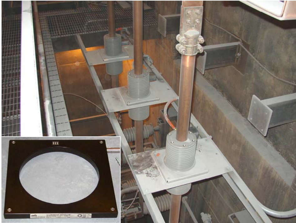
Figure 20. EAF Transformer Primary Side Rogowski Coils
