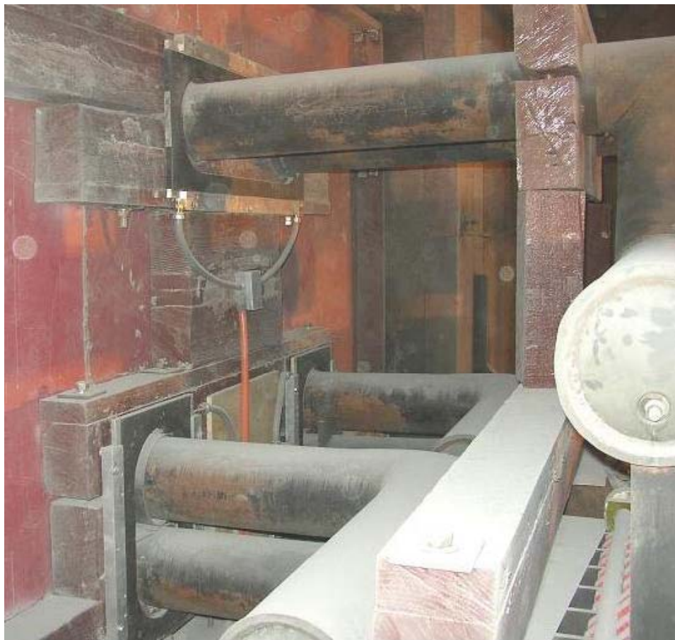
Figure 21. EAF Transformer Secondary Side Rogowski Coils
