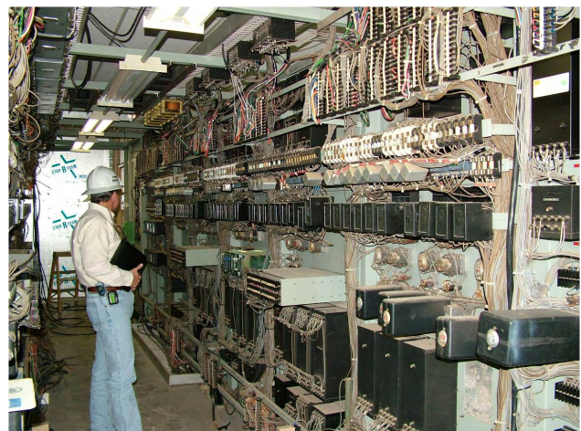
Fig. 4. Electromechanical relay panel with rear-panel wiring. This photo is courtesy of Oncor.
