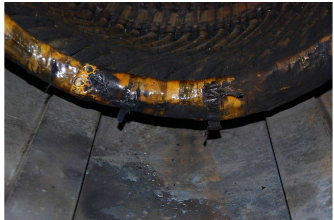
Fig. 43. Generator Fault Damage
