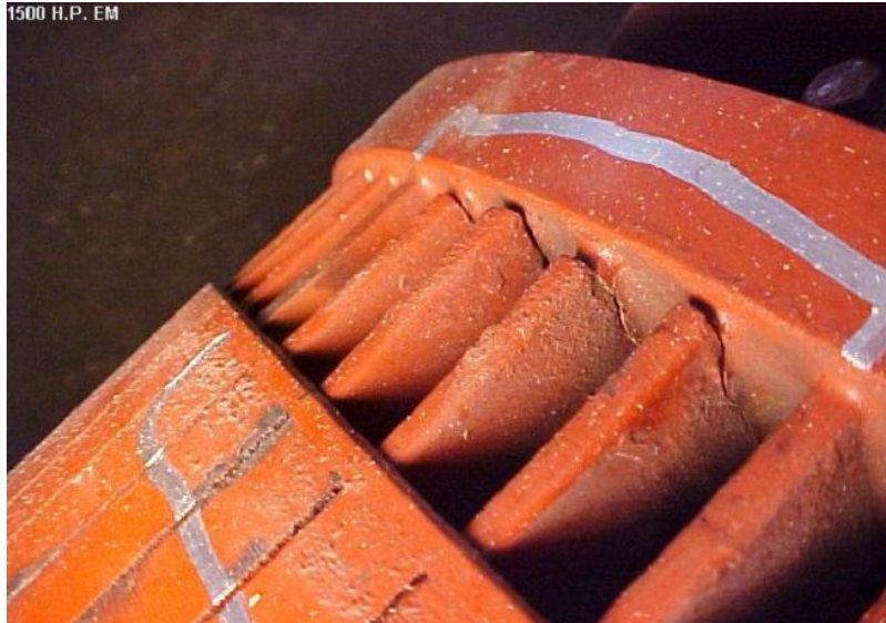
Figure 2. 6600 V, 1500 HP fan motor with broken rotor bars (field picture)
