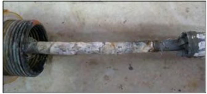
Fig. 18. A failed FO splicing box showing the rusted stand broken from the base and aluminum tube corrosion that caused pressure on fiber, high-signal attenuation, and failure of the communications system
