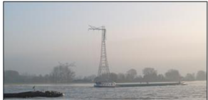
Fig. 45. Tower and feeder damage from impact of large helicopter (photo source unknown).
