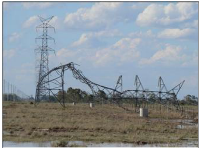
Fig. 46. One of seven collapsed towers resulting from a storm cell—OPGW was stretched but still operational
