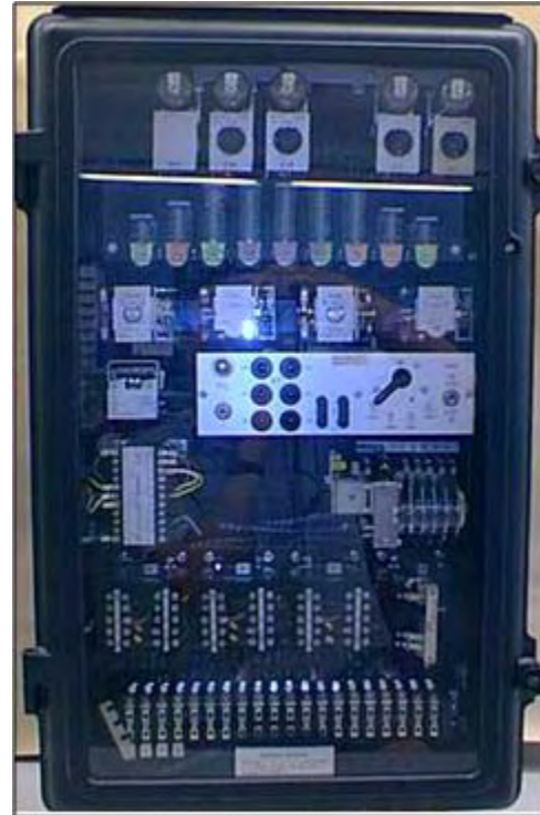
Fig. 30. First generation (electromechanical) protection relay
