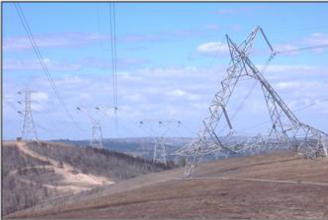
Fig. 48. Collapsed tower resulting from a major bush fire—GW was intact. (No fibers in GW)
