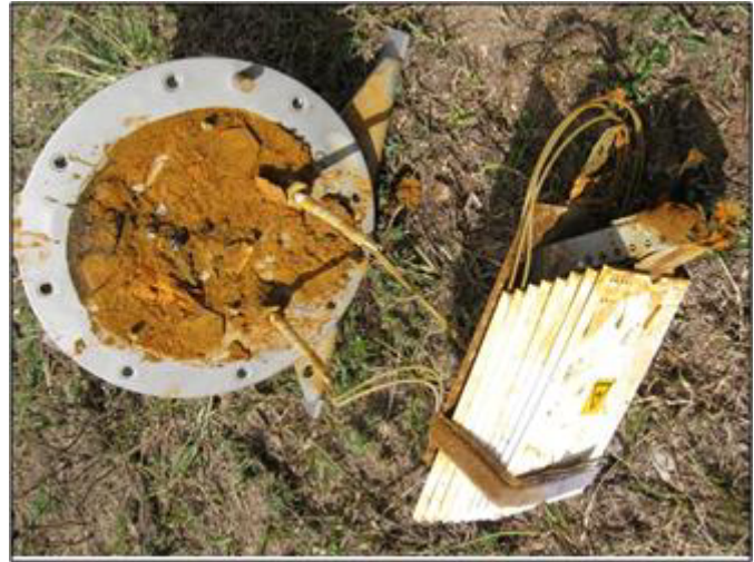
Fig. 44. A failed FO splicing box showing that the rusted stand has broken from the base
