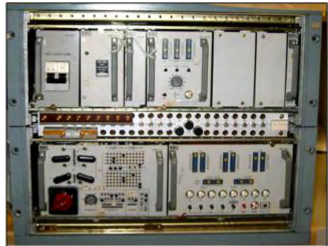
Fig. 31. Second generation (solid state) protection relay
